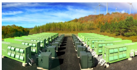
Invenergy's Grand Ridge storage facility
